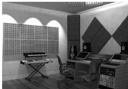
Eight RD Diffuser diffusers are bolted together and hung on the wall to create ambience in the studio.
